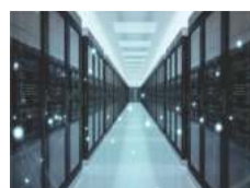
Small and medium-sized data center
