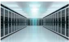
Large-scale server room
