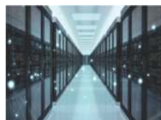
Small and medium-sized data center
