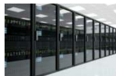
High heat density data center
