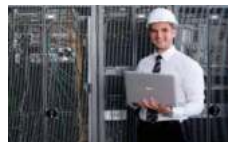
Traditional Server Room
