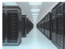
High heat density data machine room
