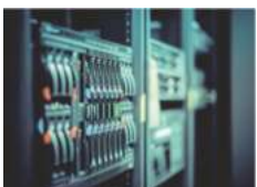
Container data center
