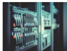
Container data center
