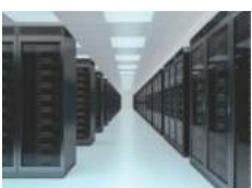
High heat density data machine room
