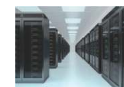
High heat density data machine room
