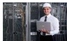
Traditional Server Room
