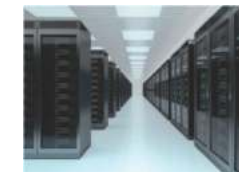
High heat density data machine room
