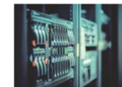
Container data center
